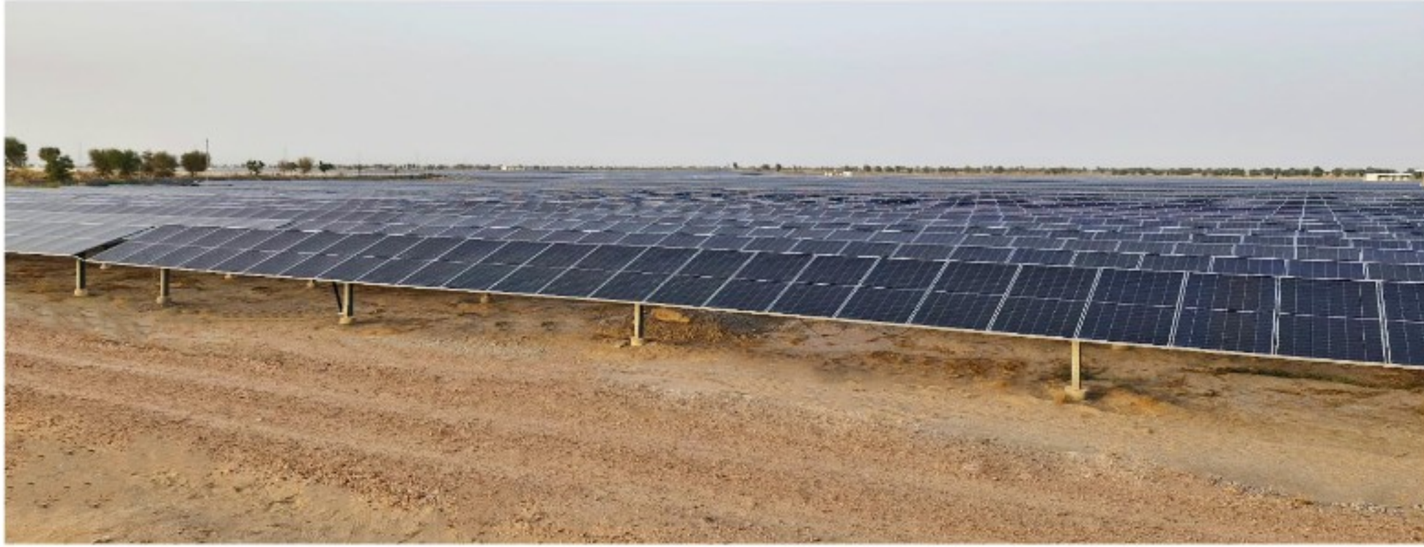
52MW - KADAPA, ANDHRA PRADESH (NSL RENEWABLE CPP PVT. LTD.)
